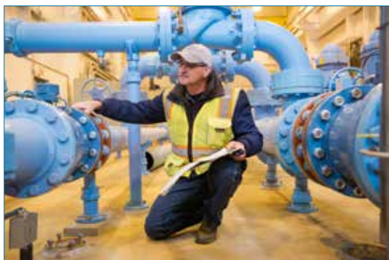
SWA Operator, Dan Roller Checks Out the Water System Photo Credit: Kyle Martin Photo
