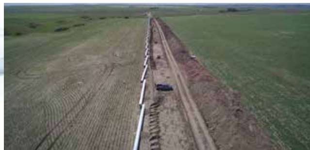
Construction of paralleled main transmission line from Lake Sakakawea to the OMND WTP
